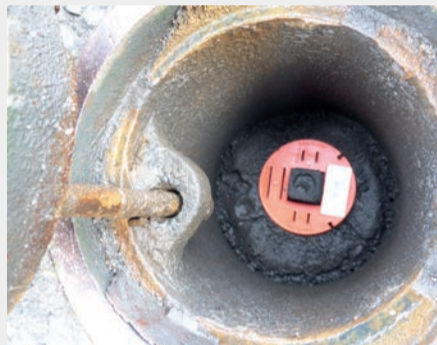
Additional information sticker „Hydrant“
