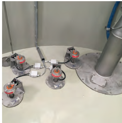
Electric position indicators made of stainless steel in a drinking water system
