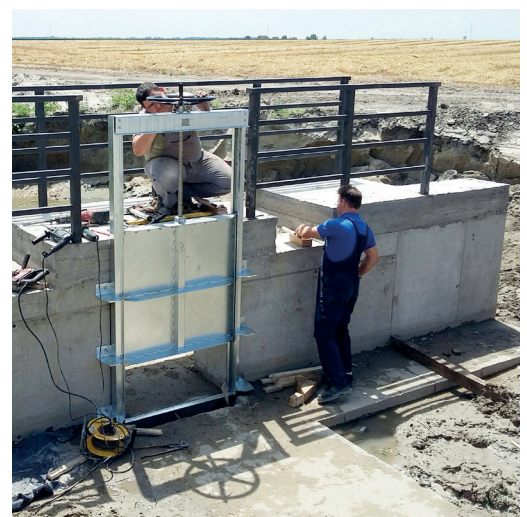
Irrigation system in Croatia, penstock 1000 x 1000 mm
