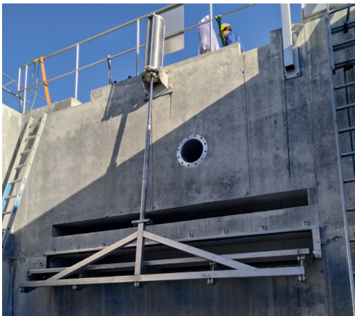
Rotary weir with front control with pneumatic cylinder, Switzerland
